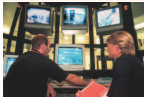
Honeywell incorporates Lantronix's SecureBox SDS1100 into its Enterprise Buildings Integrator architecture, such as in the prison security system shown here.
