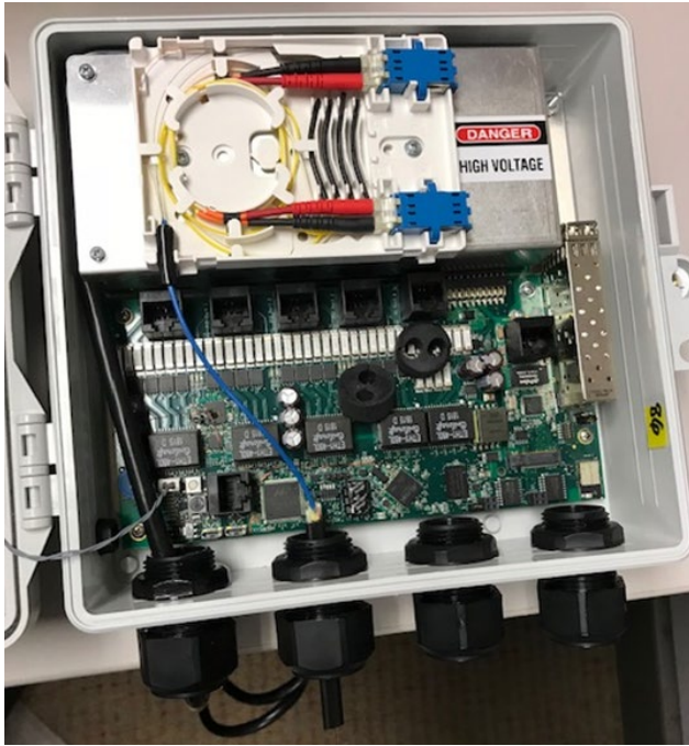
Fig. 5: Fiber Tray with Fiber (Installed)
